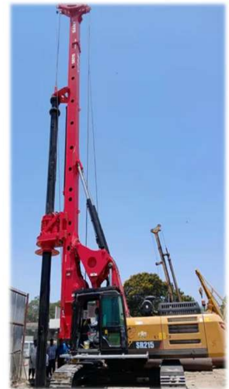
INTEGRATED EFFLUENT TREATMENT PLANT HPCL – VRMP -VISAKHAPATNAM
