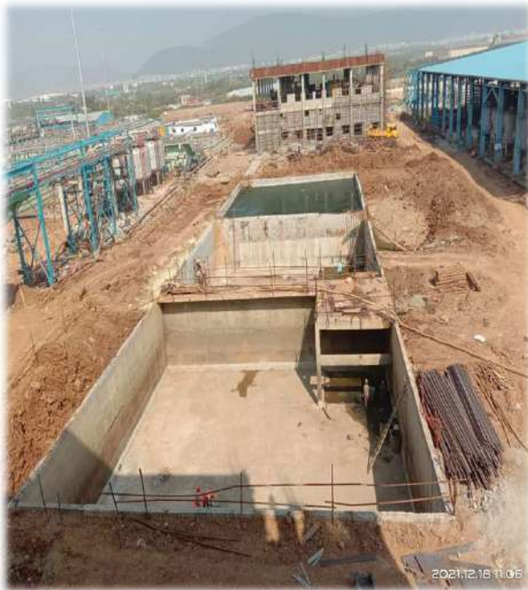
DM-V PLANT (DMP-V) & SWORE-II DESALINATION PLANT EFFULENT DISPOSAL SUMP – HPCL- VRMP VISAKHAPATNAM – ANDHRAPRADESH - INDIA
