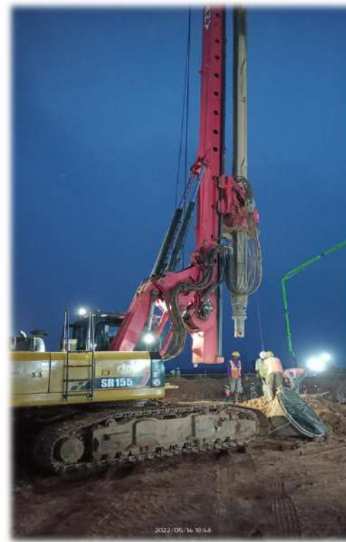
CRUDE & VACUUM DISTILLATION UNIT – HPCL- VRMP VISAKHAPATNAM – ANDHRAPRADESH - INDIA
