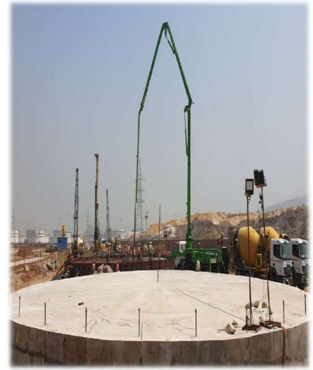
Equalization Tank Pad – IETP- HPCL – VRMP VISA KHAPATNAM – ANDHRA PRADESH - INDIA
